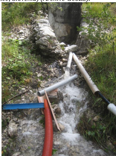
Obrázek 4: Example of inappropriate implementation and maintenance of drainage system caused that surface water flows uncontrolled along the landslide and across the road (spring Urbas, landslide Urbas, Jesenice)..
