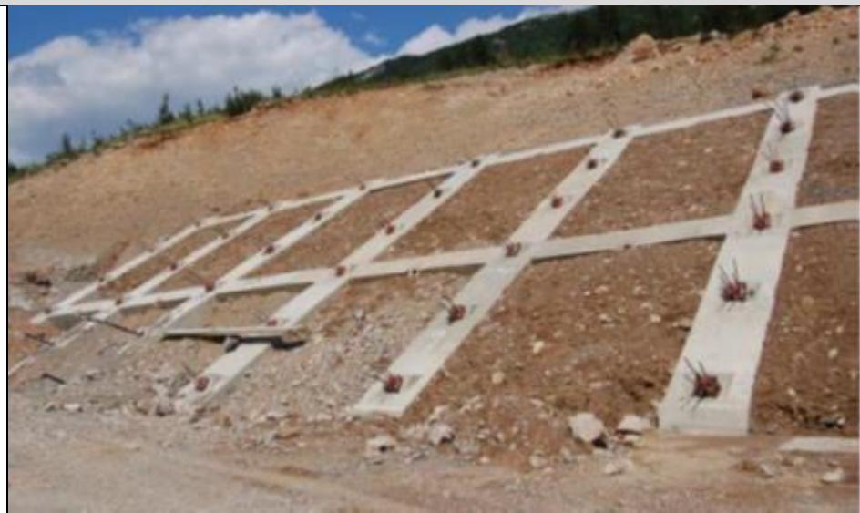
Figure 10. Anchored reinforced concrete frame on highway Razdrto-Vipava (landslide Rebernice, Slovenia) (photo B. Pulko).
